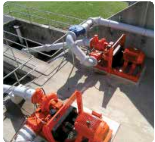
Permanently installed electric drive Dri-Prime pumps moving effluent from a secondary trickling filter to a chlorination chamber and then discharge.
